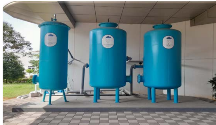
Rainwater filtration units, India
