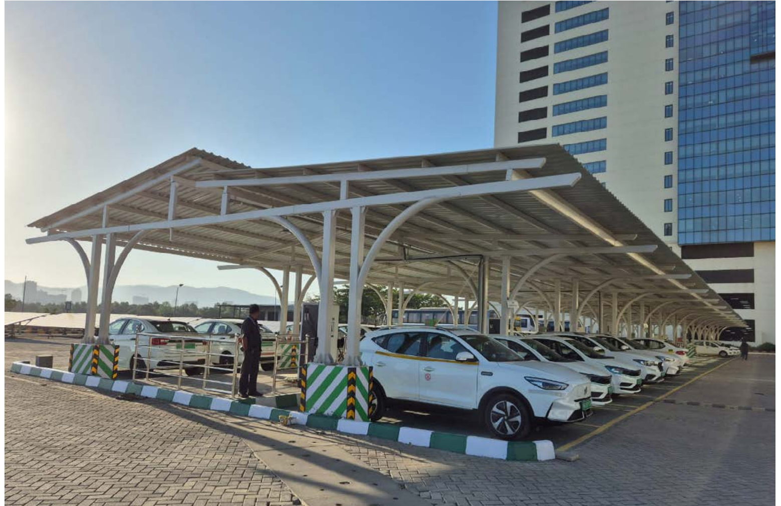
EV charging station, Mumbai, India
